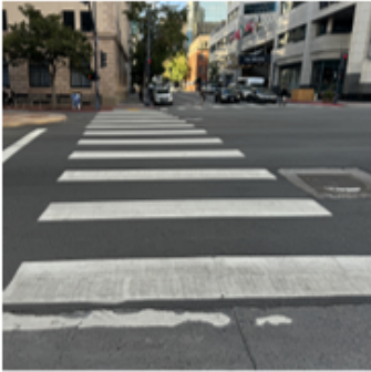
Continental Crosswalks improve crosswalk visibility and are known to improve driver yielding compliance.
